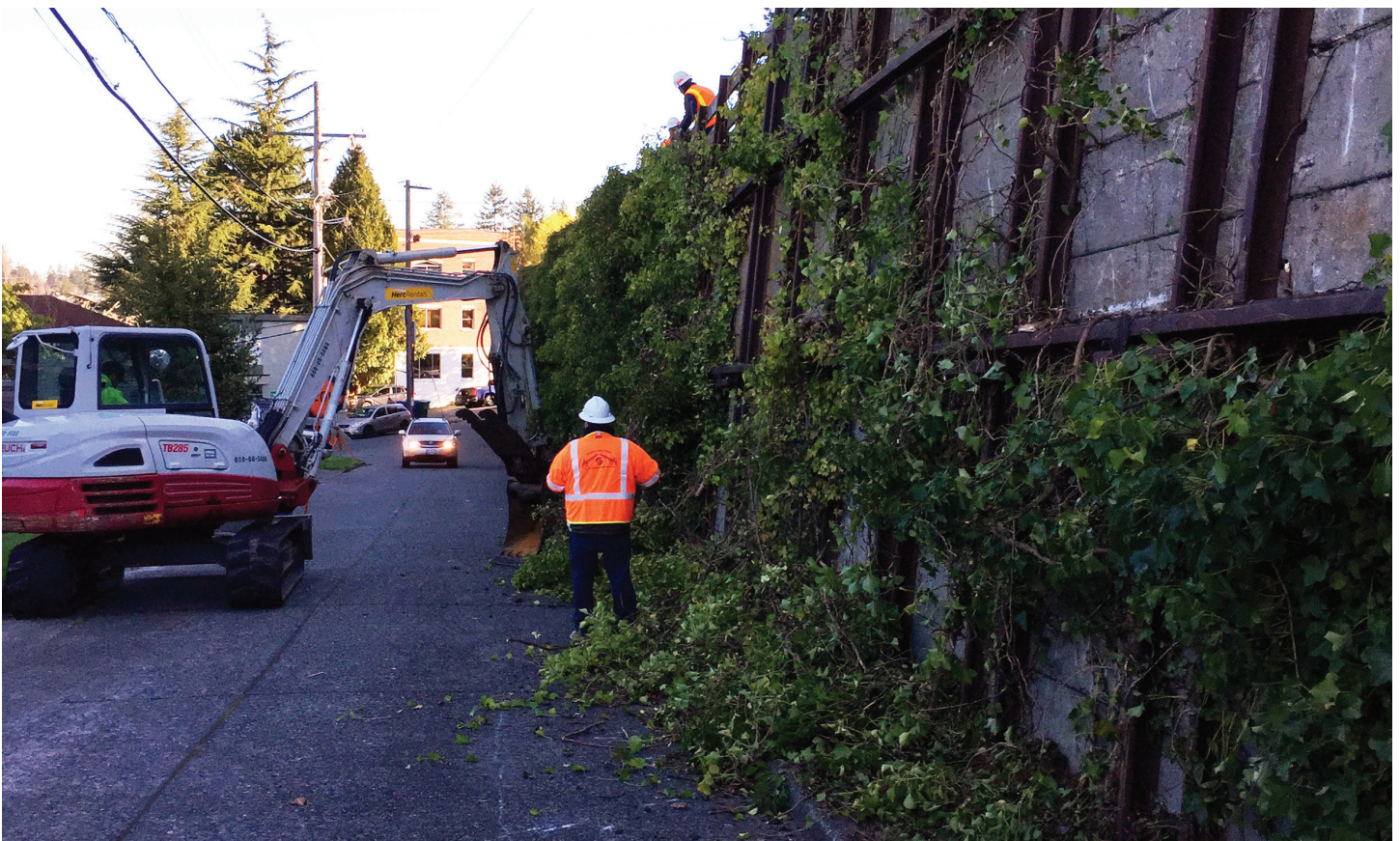
Inspection at retaining wall on 44th Ave SW, between California Ave SW and SW Austin St
