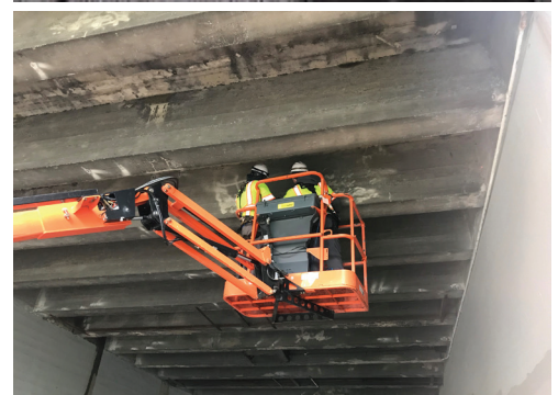
TOP TO BOTTOM: Ballard Bridge Operator; Airport over Argo Bridge Inspection; Load Testing on Phinney Ave Bridge; Emerson Seismic Join Grating Replacement
