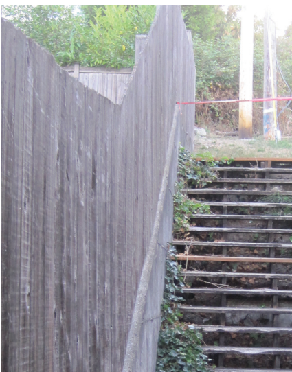
SW Willow St between California Ave and 42nd Ave SW after replacement
