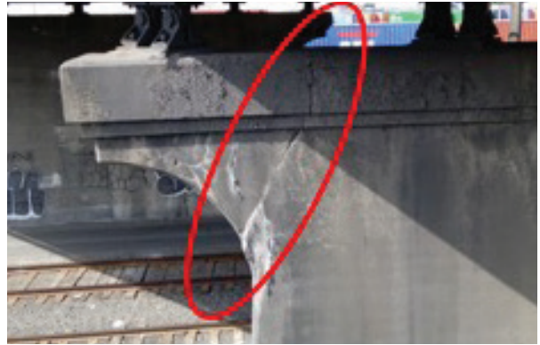
4th Avenue South Bridge: Cracked cantilevered bridge pier section over the Argo Rail Yard
